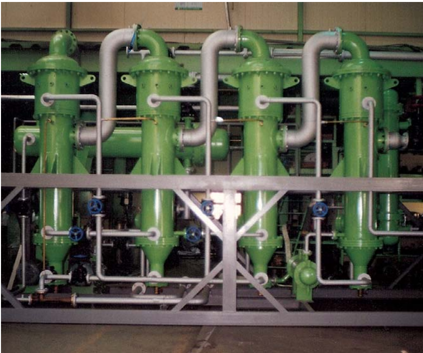
▲ We have developed the design and manufacturing technology of four effect type desalination system ; joint KIMM
