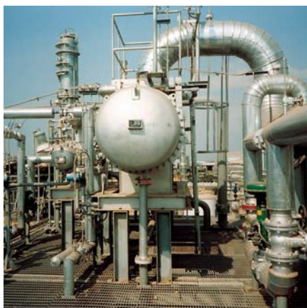
2 stage steam jet vacuum system with pre-condenser for crude oil refineries : TPI phase III
