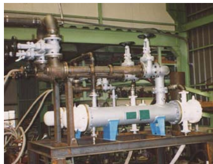
Two elements 2 stage steam jet ejector with surface condensers for power plant : Co-generation plant
